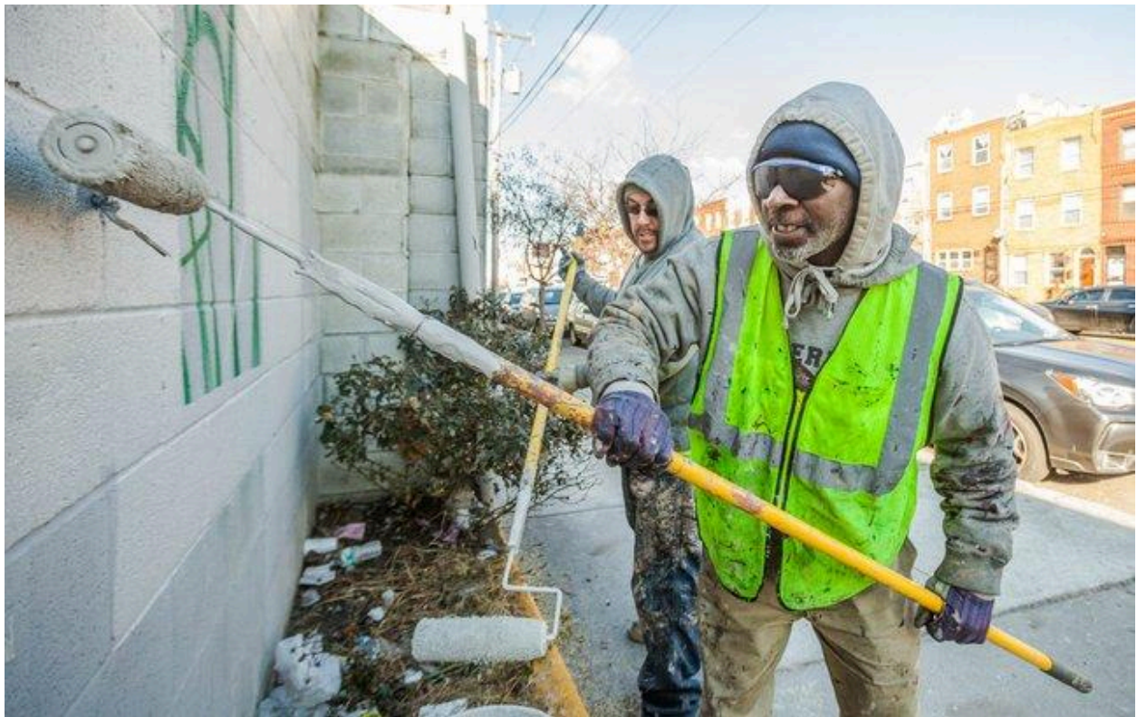
CLIP's graffiti abatement employees paint over graffiti tags at the corner of Sixth and Washington streets. Graffiti removal is a free service for residents and businesses in Philadelphia. 13
